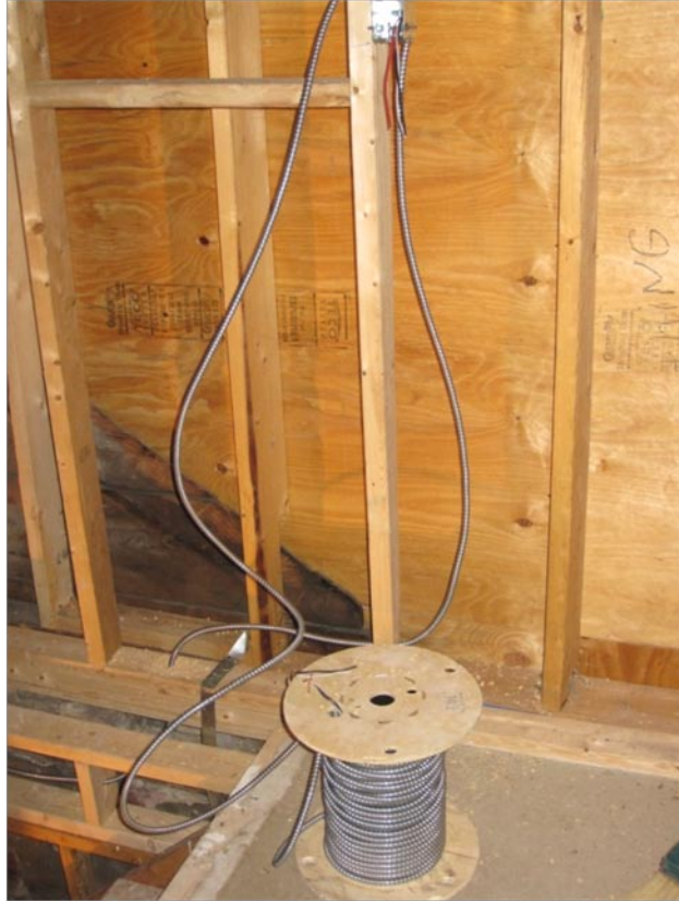
Photo 5: BX armored cable installed throughout the house.
