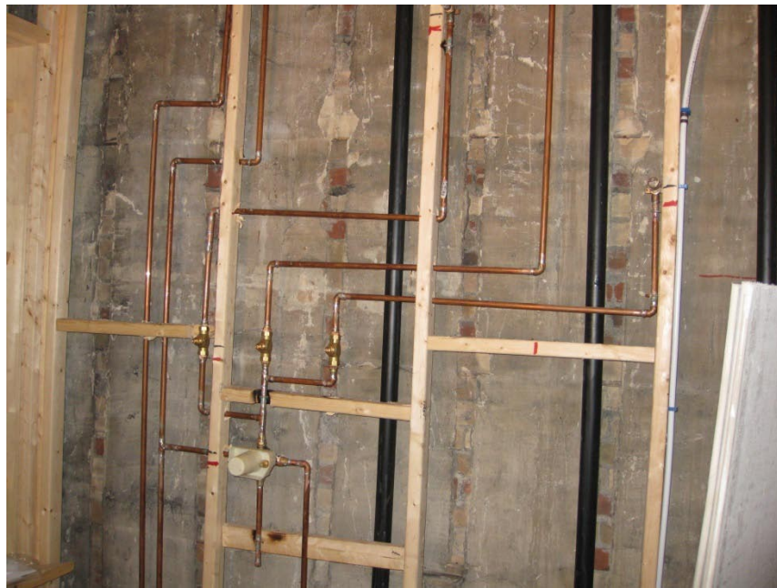
Photo 6: Copper plumbing for hydronic underfloor heating system.
