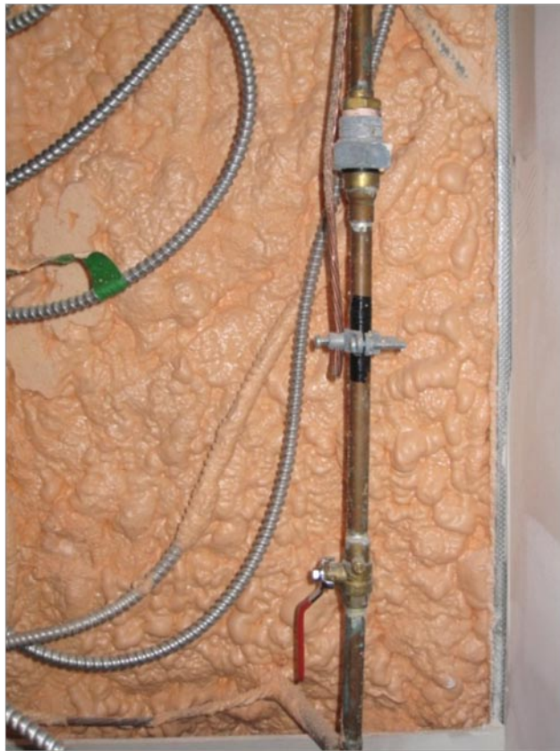
Photo 4: Dielectric coupler installed on plumbing system.
